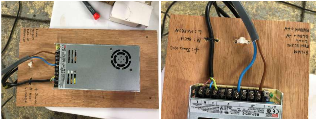
Detail of the power supply included with the installation
